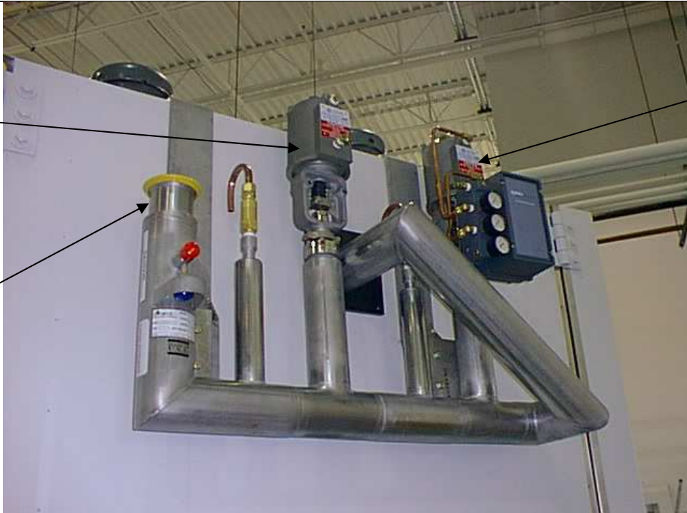
3 - REAL-36 & 48 LN2 control valves.
