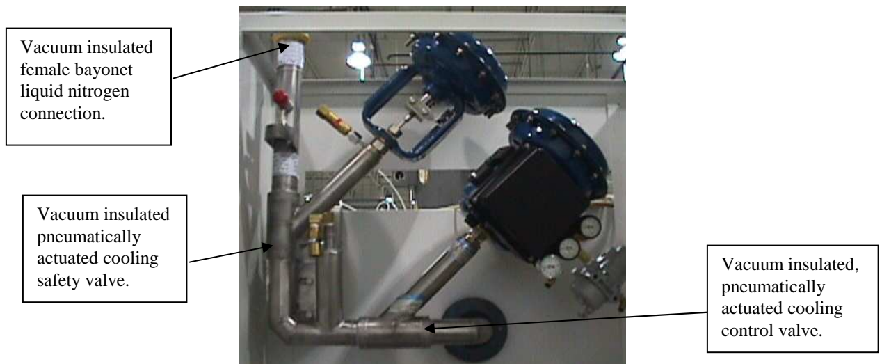
2 - REAL-30 LN2 control valves.
